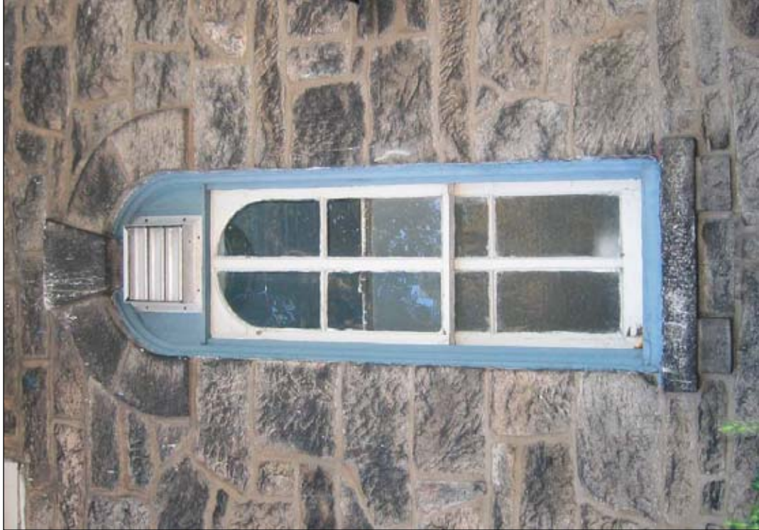
Figure 52: North elevation. Detail of window with addition of metal exhaust fan. Stone surface soiling is also visible, especially on the keystone arch and sill.
