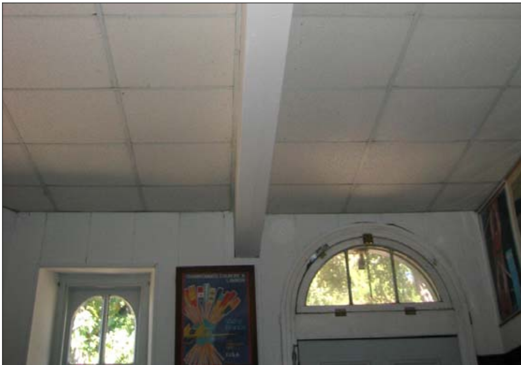
Figure 47: Front meeting room, north wall. View showing sheathed steel beam where interior load-bearing wall once stood. Photo also depicts suspended ceiling.
