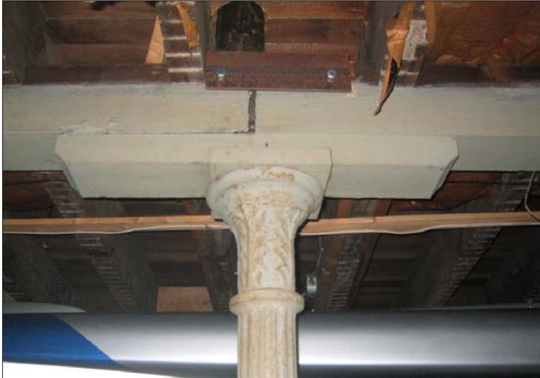
Figure 48: Basement, looking eastwards. View of cast iron fluted column and ceiling joist. Wood shows signs of rotting deterioration.
