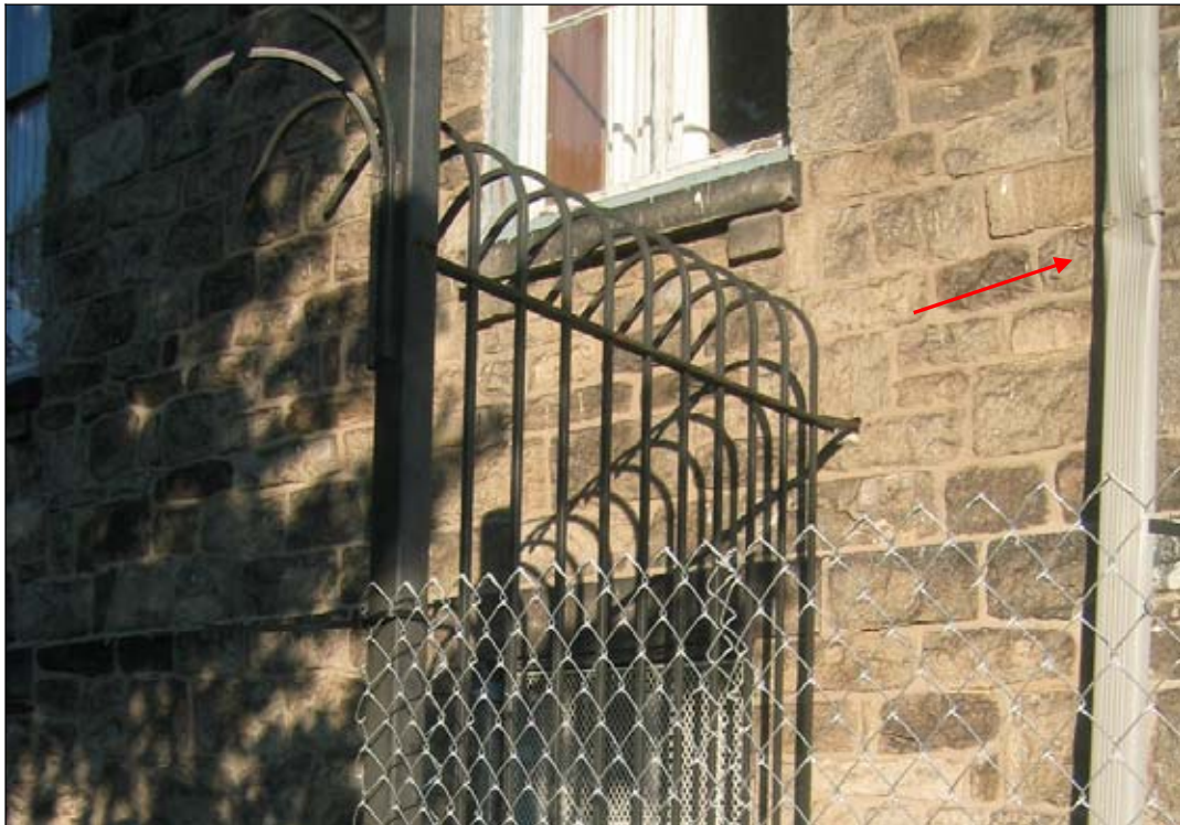
Figure 53: West elevation. Detail shows crushed aluminum downspout which may impede water flow during heavy downpours.
