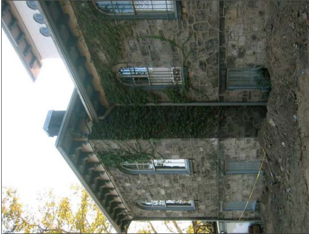
Figure 50: East elevation, looking south towards the river. View shows vegetation in the form of ivy on the wall surface.
