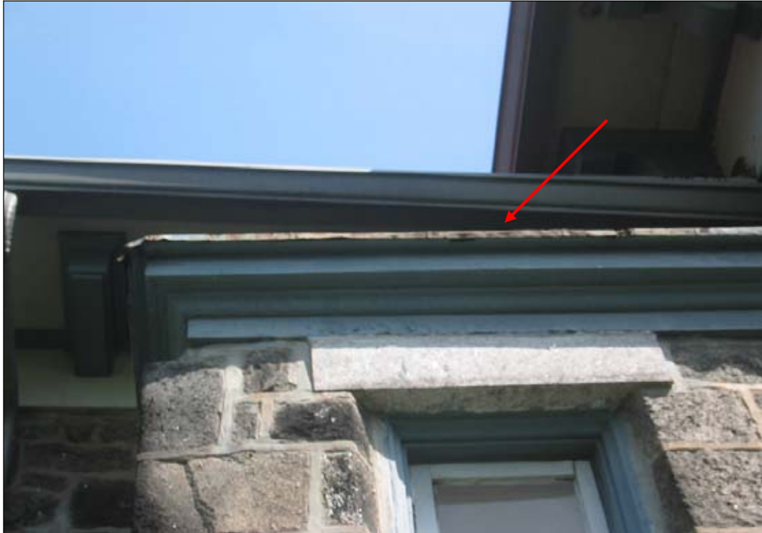
Figure 54: West Elevation, detail of roof. View shows rusting flashing along edge.
