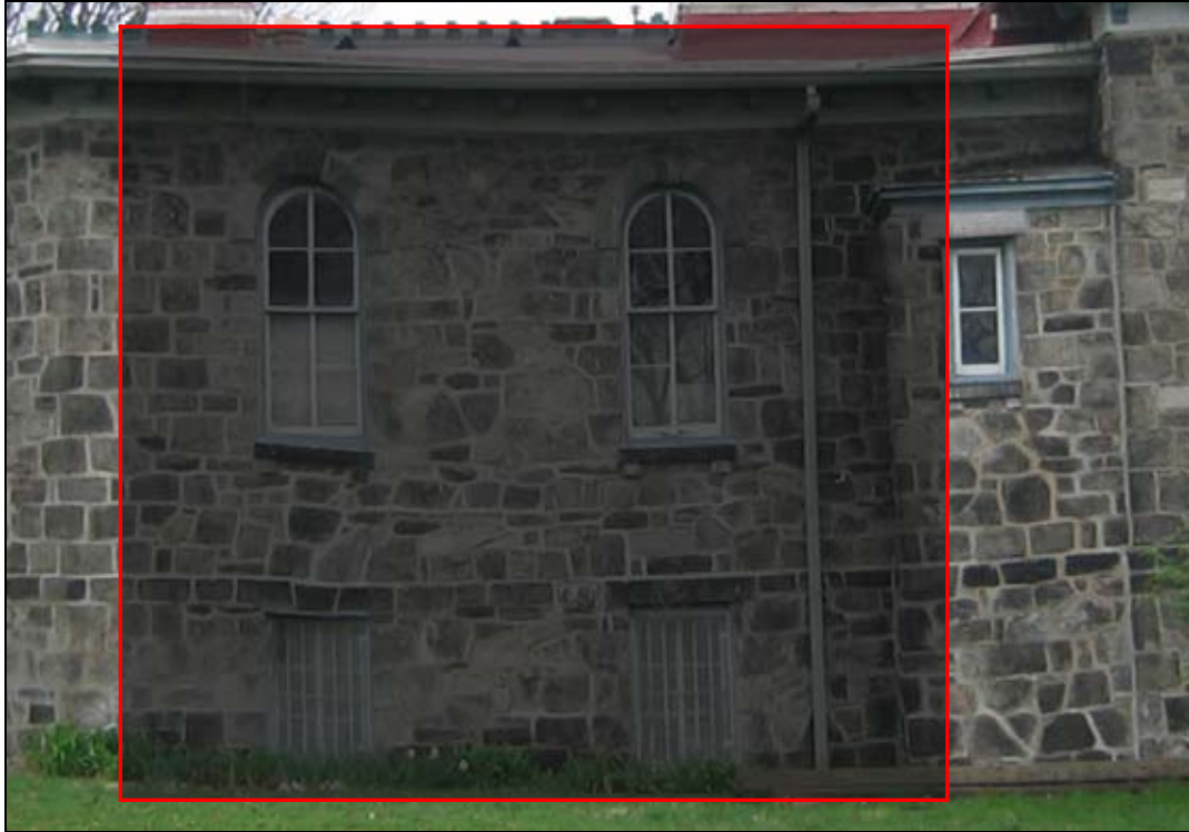
Figure 42: West elevation. View lateral showing wall displacement, especially in the marked area. (Photograph by author, 2005) 1
