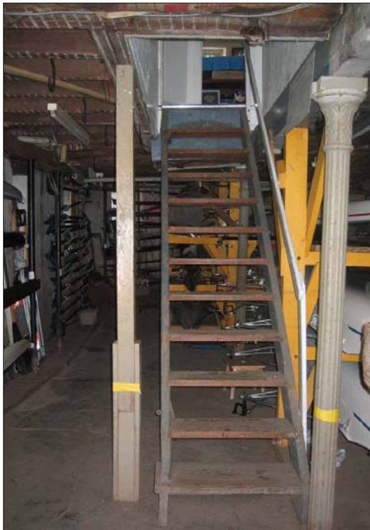
Figure 18: Basement with stair and columns - both wooden and cast iron, view looking north. (Photograph by author, 2005)
