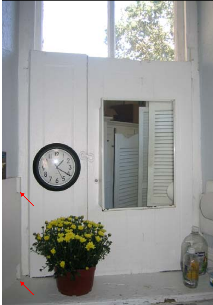
Figure 19: Shower/Bathroom, north wall. Detail of historic interior shutters. Arrows point to the notches where bars were slipped into place for security purposes. (Photograph by author, 2005)
