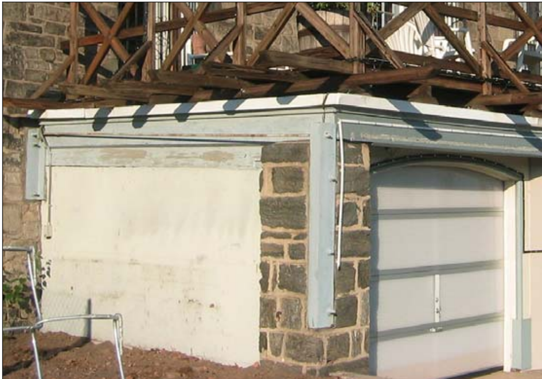
Figure 45: West and south elevations, detail. View showing bracing units on back enclosed porch.
