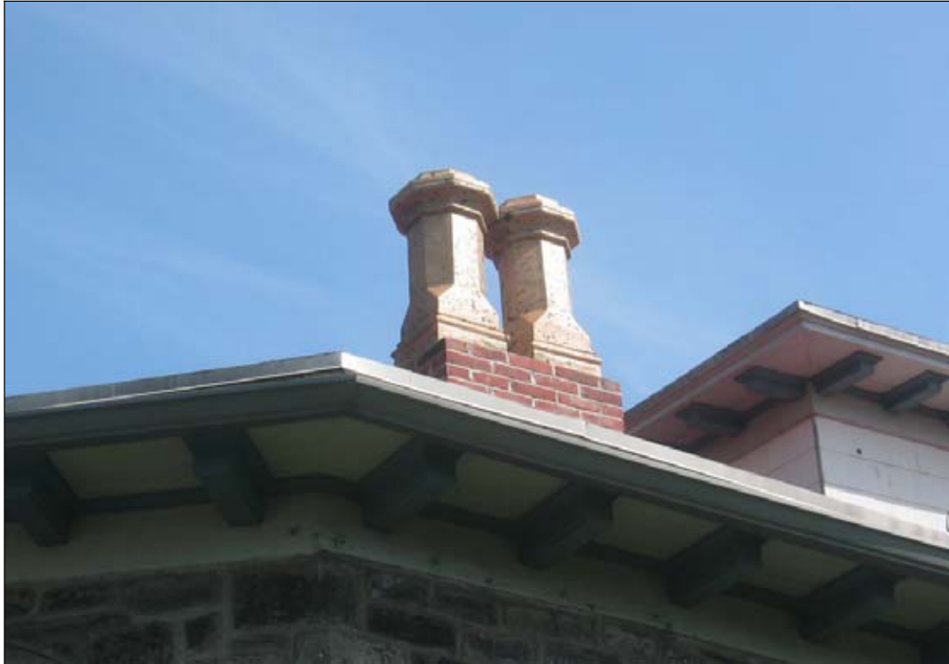
Figure 56: West elevation, detail of roof. View shows flaking paint on terra cotta chimney stacks.
