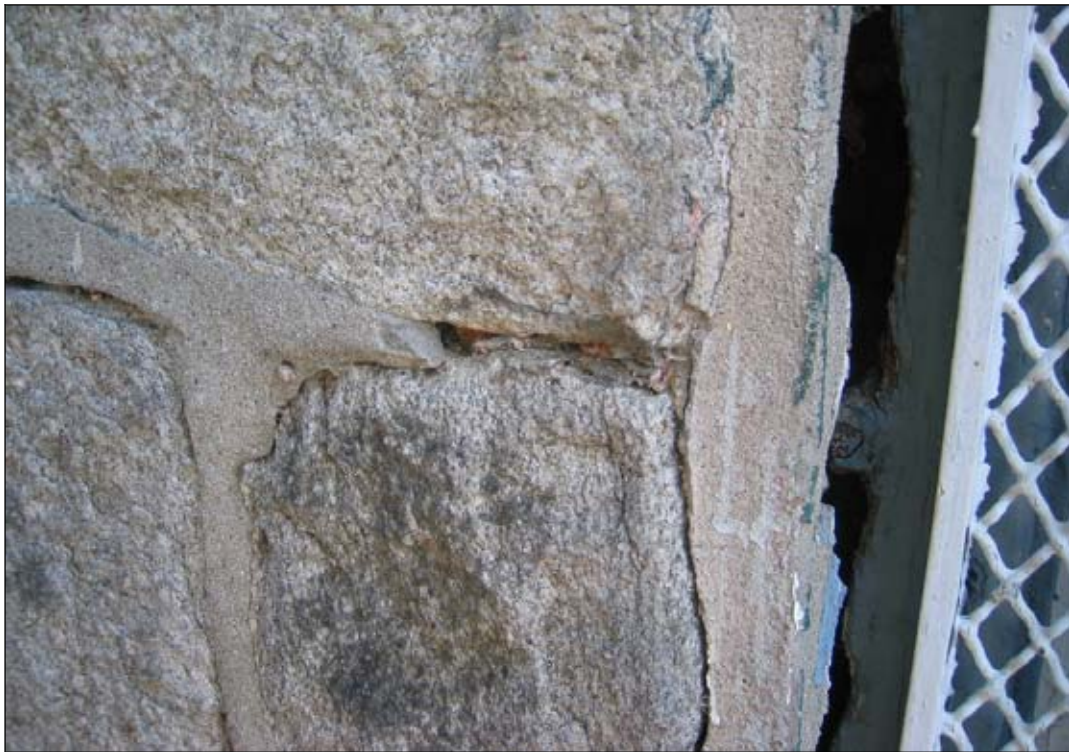
Figure 51: West elevation, detail. Loose and missing mortar from around rough window opening.
