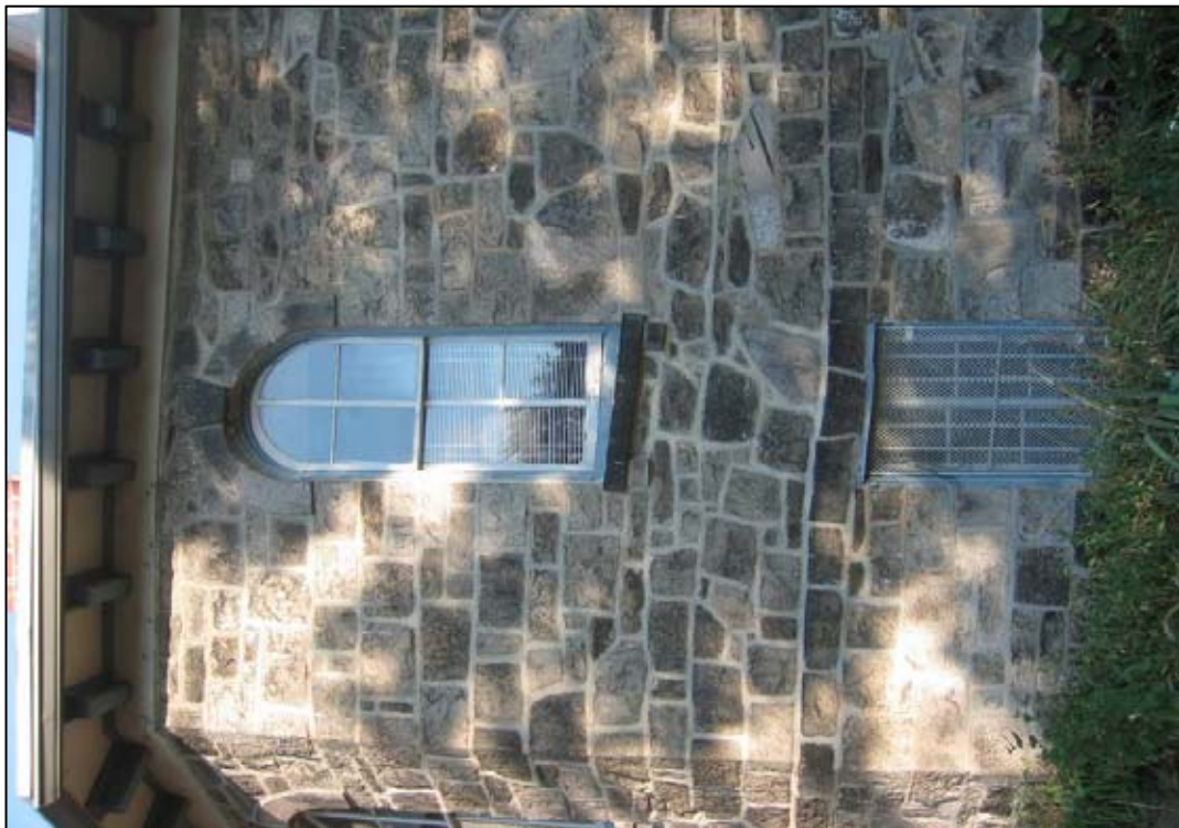
Figure 43: West elevation, detail. View showing window distortion.
