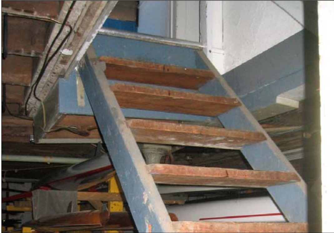
Figure 15: Basement stair, old stinger and new treads visible, along with original stair opening and platform. (Photograph by author, 2005)
