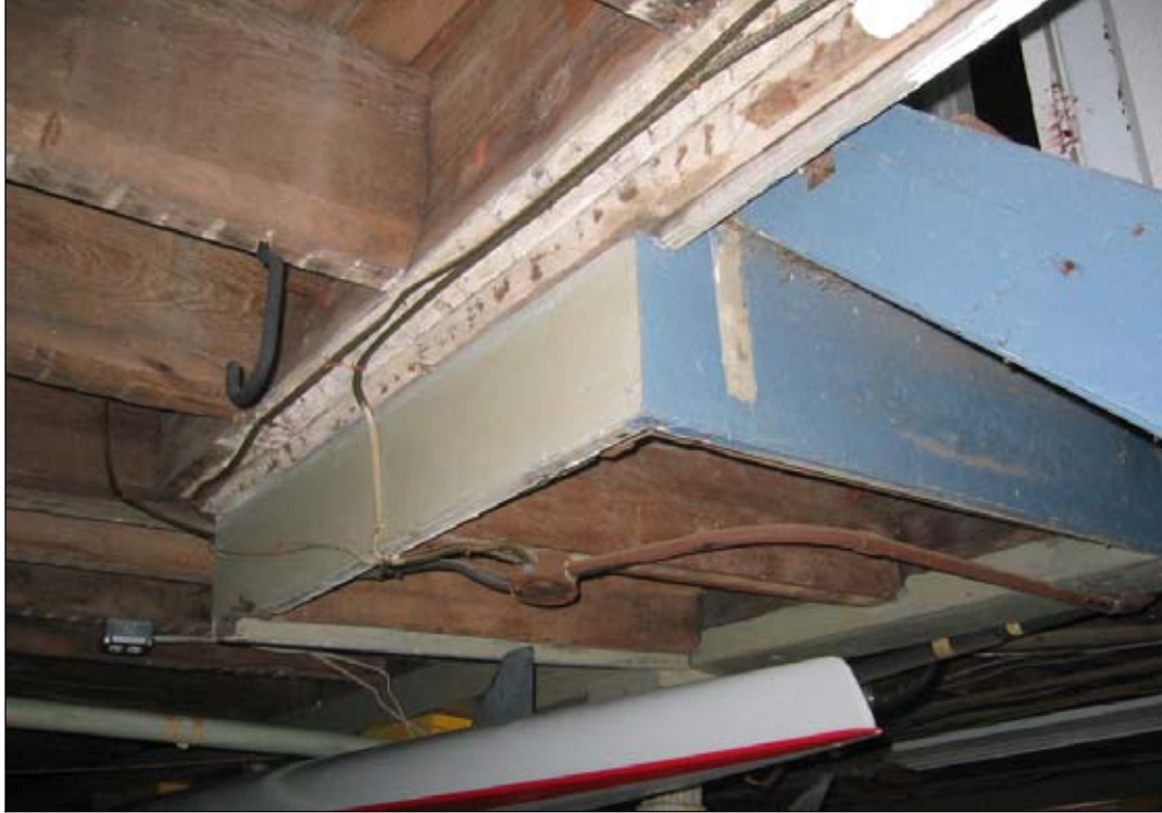
Figure 60: Basement, ceiling detail beneath stair opening. View shows remnants of old electrical wiring, along with newer additions.
