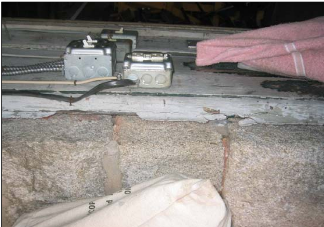
Figure 59: Basement, beside back bay door. Detail shows examples of modern light switches and power outlets.
