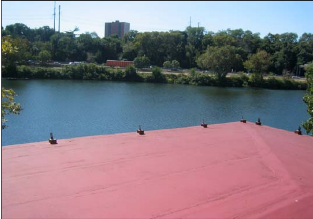
Figure 24: Main roof, looking south towards the Schuylkill River. The shallow surfaces are where water gathers into ponds, thereby increasing the potential for leakage and failure. Evidence of the balustrade appears along the roof edges. (Photograph by author, 2005)
