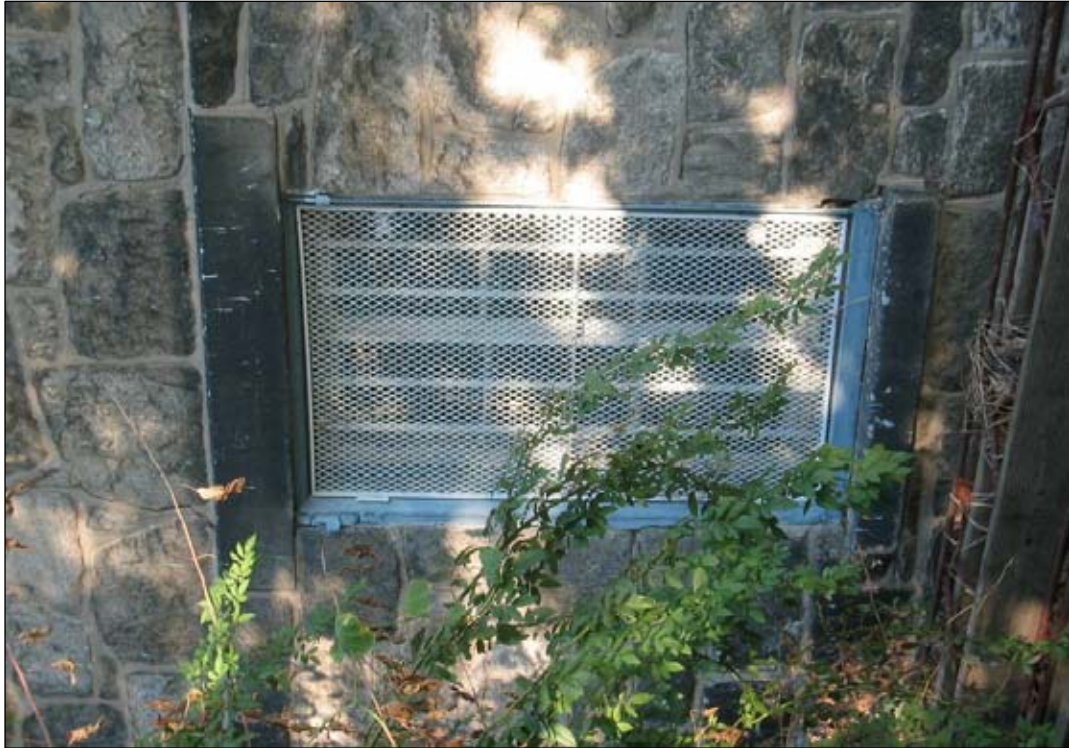
Figure 58: West elevation, detail. View show metal rods and grille over basement window opening.
