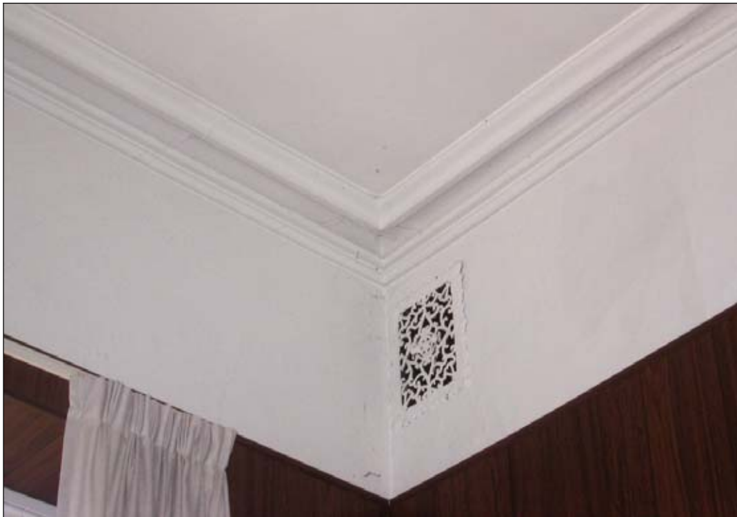
Figure 55: South meeting room. Detail shows ceiling wall diffuser.
