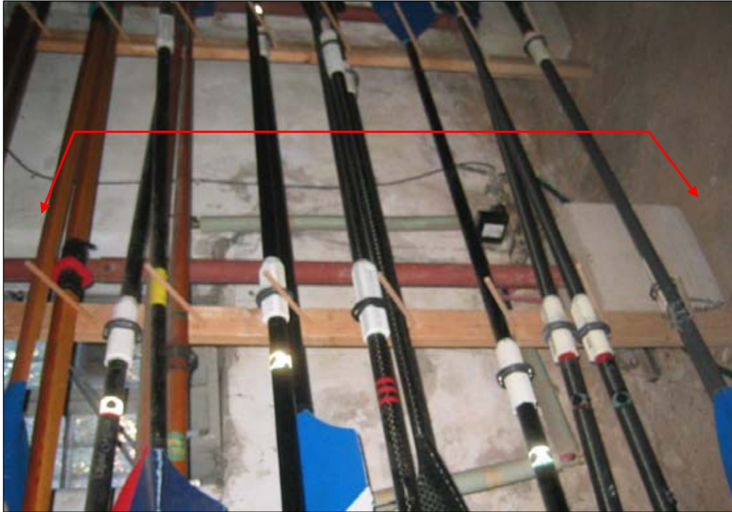
Figure 46: Basement interior, west wall. View showing scaffold jacks holding up wall and floor above.
