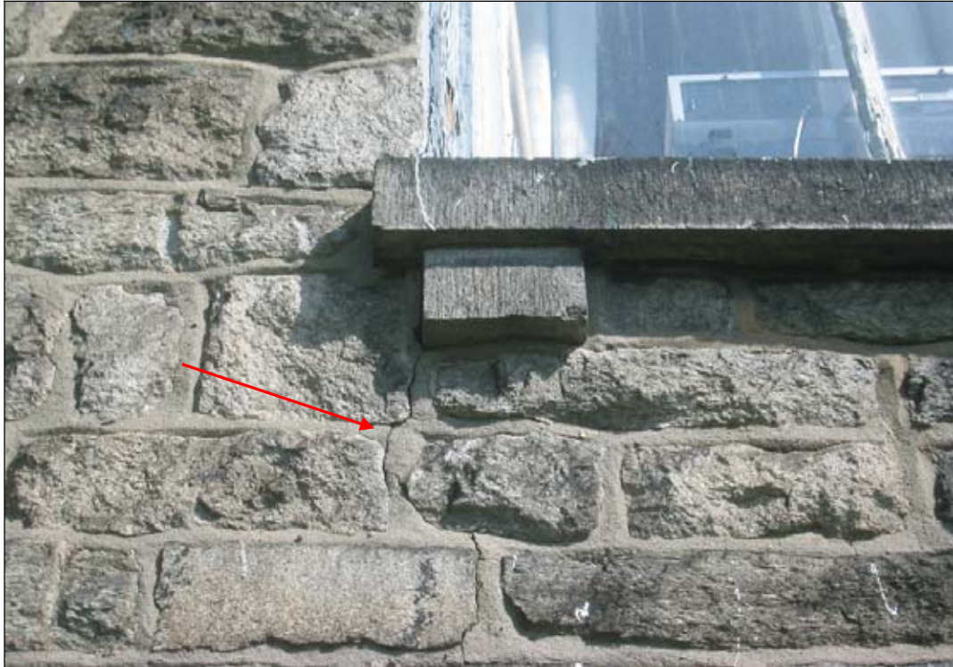
Figure 44: West elevation, detail. Evidence of cracking in mortar beneath window corners.
