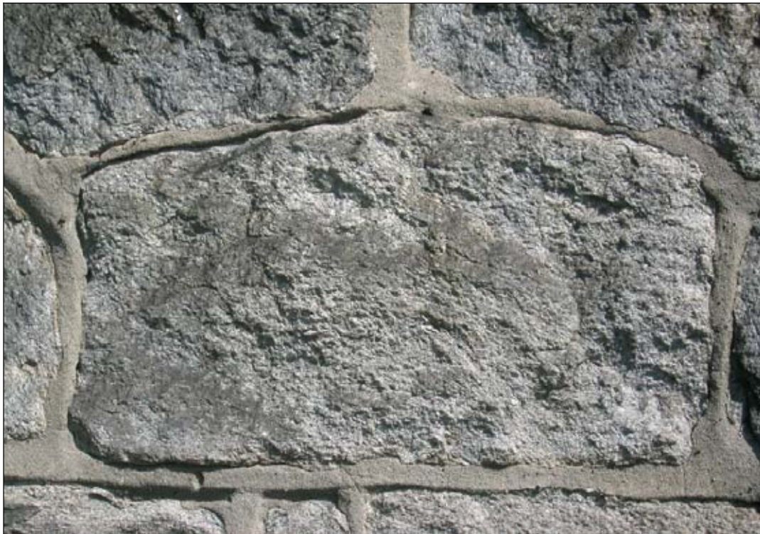
Figure 22: West elevation, detail of building's masonry, coarse-grained and soiled granite. (Photograph by author, 2005)
