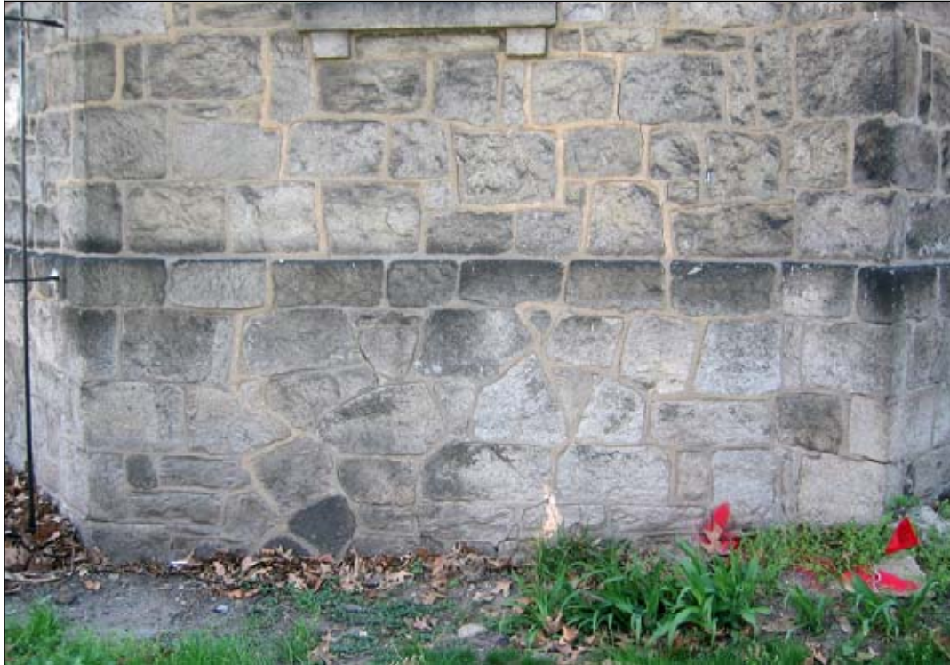
Figure 21: Northwest elevation, detail showing soiled stone, especially along the stone articulation separating the raised basement and first floor and on the building's corners. (Photograph by author, 2005)
