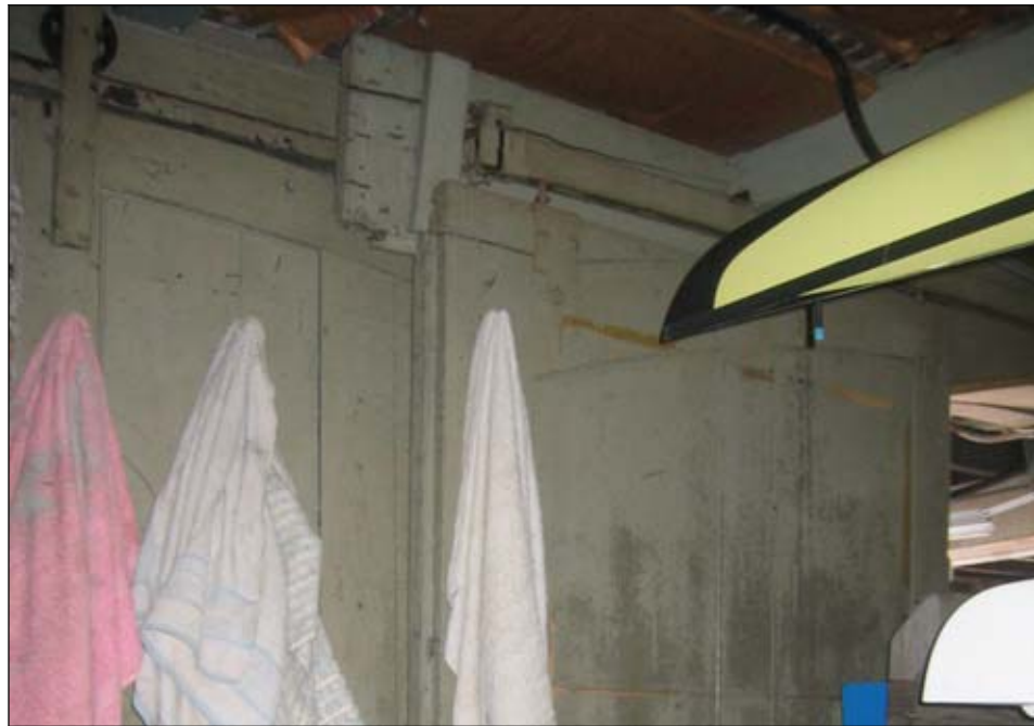
Figure 17: Original wooden doors with iron rails and rollers, basement, south wall. (Photograph by author, 2005)
