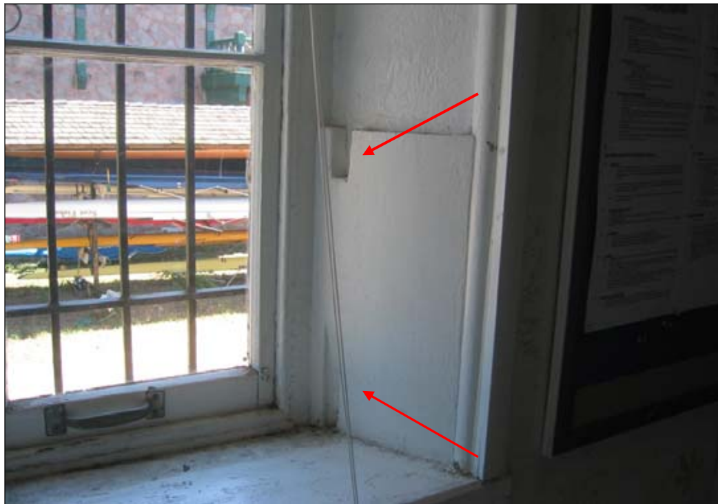
Figure 26: Locker room, east wall. Detail shows trace of shutter protection system. (Photograph by author, 2005)
